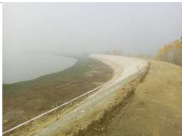
No Barricading of Site
