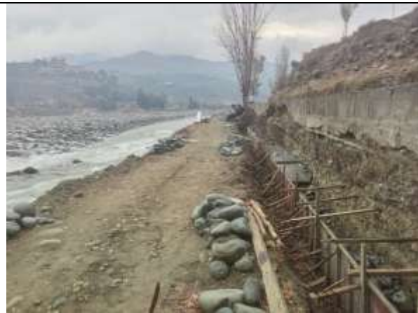
No Barricading of Access Route
