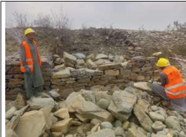
PPEs used but Damaged
