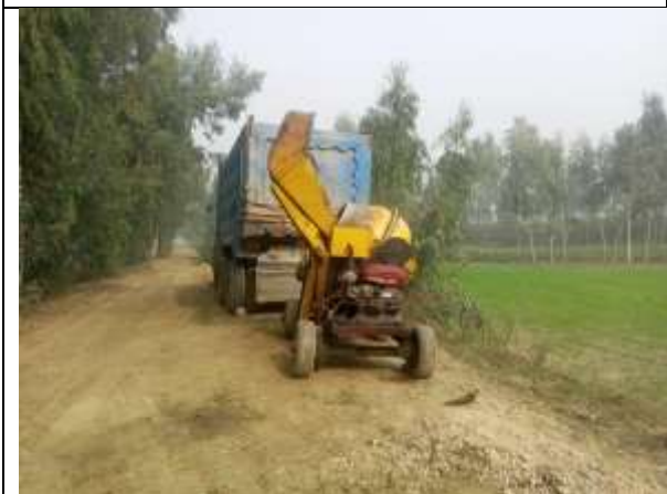
Mixer in Poor Condition
