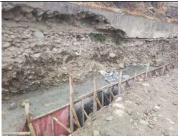
No Barricading of Site
